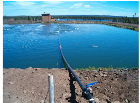
Summer operation, showing floating HDPE lateral
